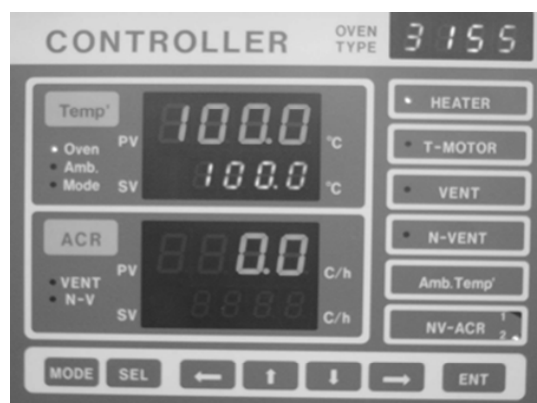
Control Panel (Temperature controller+Air change meter)
